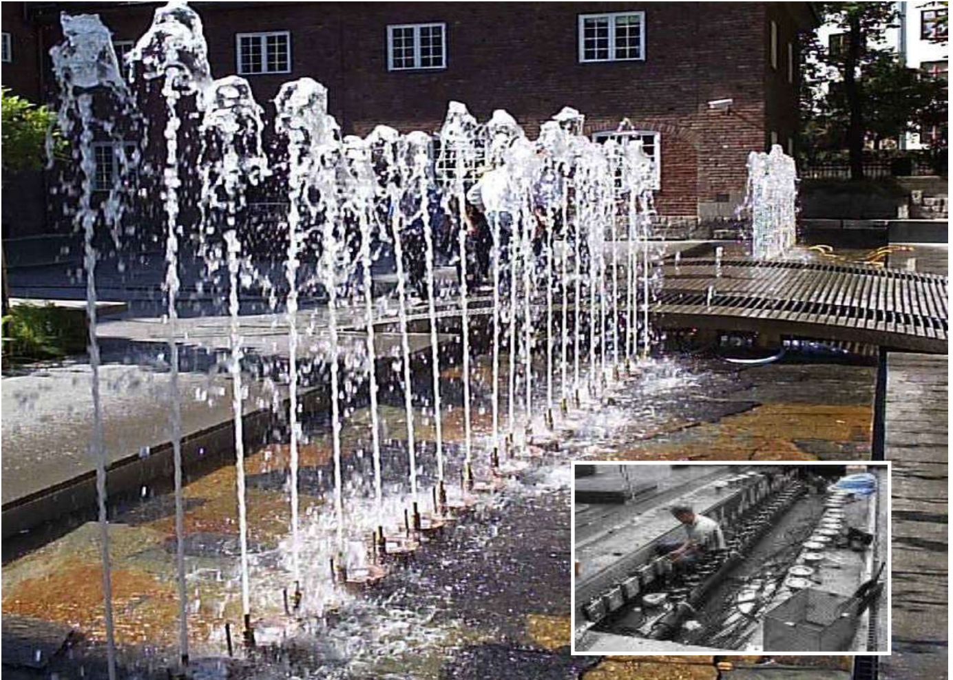
PEM 812-1 with PEM W114-1-100 Water Switches and PEM C 133-4 Submersible Lightfixtures
