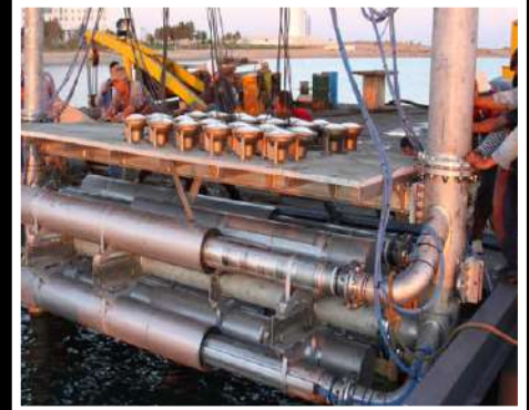
Submersible Pumps with Lights
